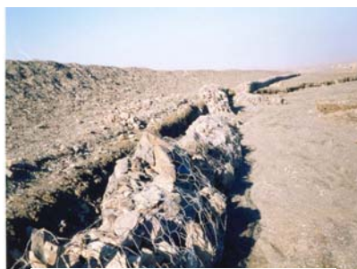
Damaged Gabions in December 2002 flooding
